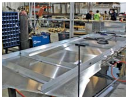
Stephen Pass, Media 1's lead fabricator, cut the interior framework from aluminum angle and attached it behind the sign face with 3M epoxy and spot welds.
