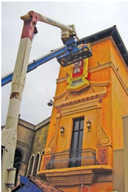
Media 1 installed the sign with a 65-ft., Altec bucket truck on a Ford F800 chassis. The final electrical hookup required approximately four hours.
