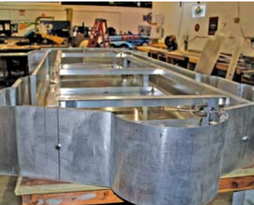
An aluminum-angle “cage” supports the structure. While fabricators installed the cage, they also created lifting points to help installation with a bucket truck.
